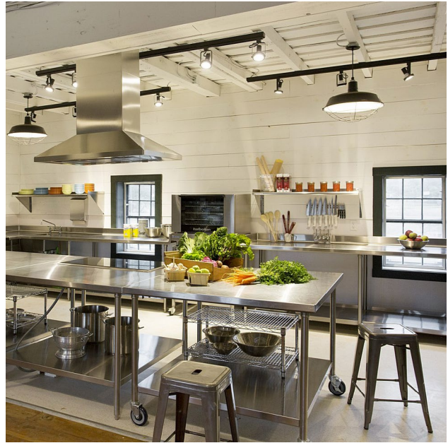
POWISSET NET POSITIVE BARN - APPLIANCES AND HIGH EFFICACY LED LIGHTING ENSURE EFFICIENT ENERGY CONSUMPTION. PHOTO: ERIC ROTH
